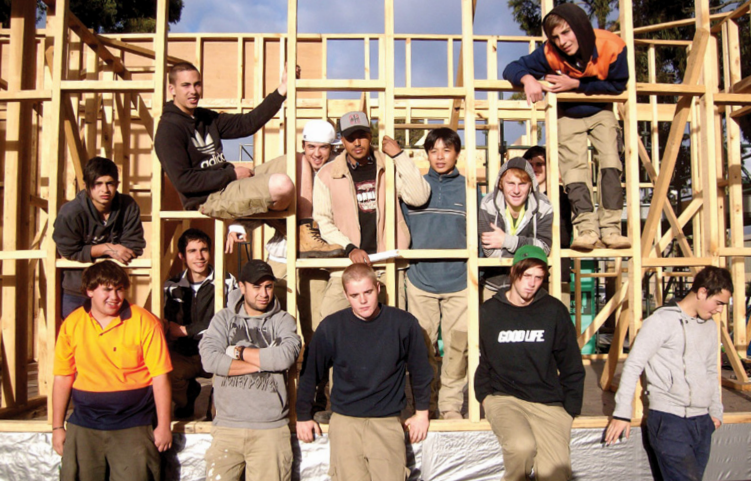
OO VU'S ASPIRING CARPENTERS: STUDENT-BUILT TRANSPORTABLE HOMES ARE BEING MOVED TO ALL PARTS OF THE STATE AS GRANNY FLATS AND BEACH HOMES.
